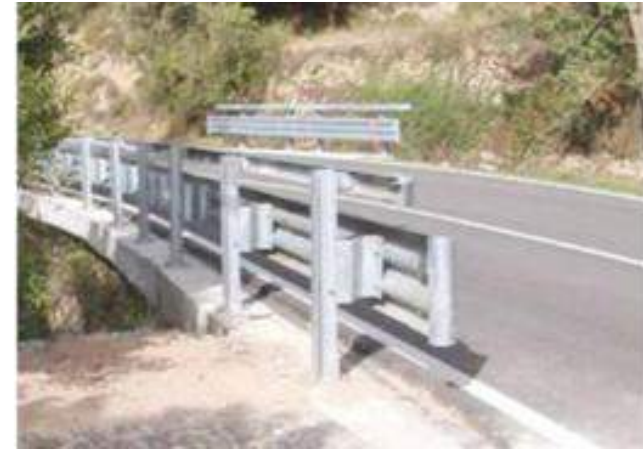
Hazardous safety barrier terminations
